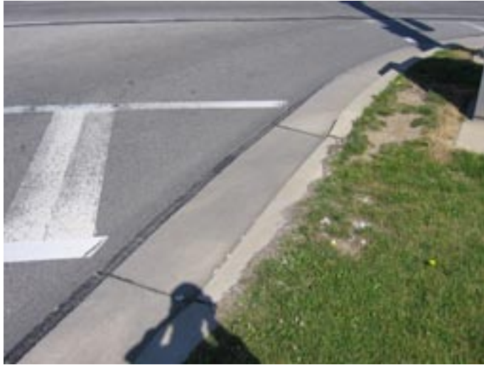
CROSSWALK AND CURB CUT WITHOUT ADJACENT SIDEWALK AT THE INTERSECTION OF HERMITAGE ROAD AND STATE STREET
